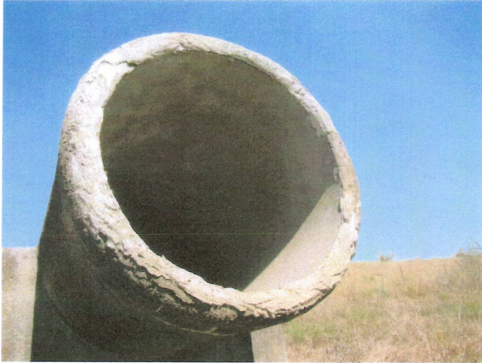
Photograph 11: Spalling at outlet pipe discharge.
