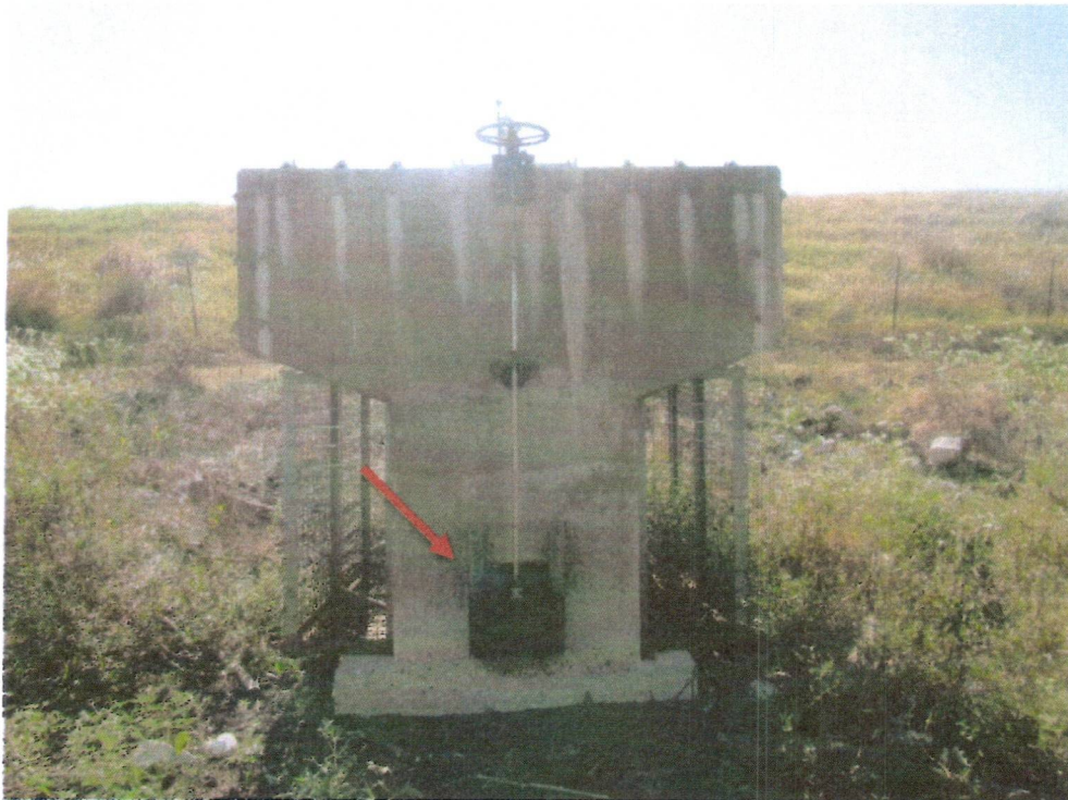
Photograph 14: Low flow outlet valve.
